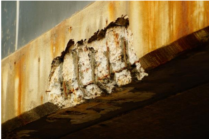
Concrete spalling on a bridge; © AdobeStock / Kay Gebauer/Wirestock
