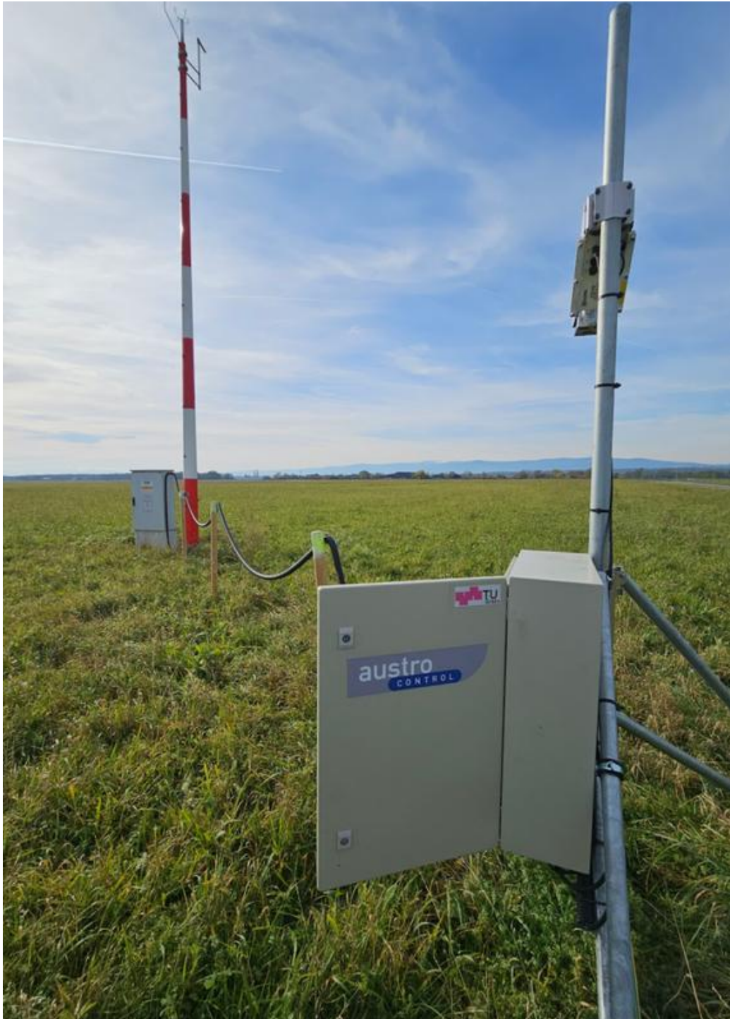
A field mill in the north of the Graz Airport site. RTLRA 2024 - TU Graz
