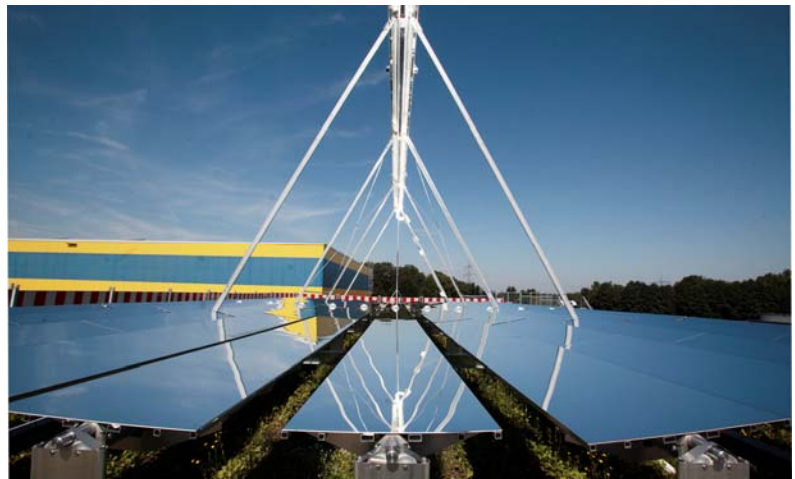
Solar thermal pilot plant in Umkirch near Freiburg, Germany. In the research project "AgroKühl", solar thermal energy is utilized to power cold rooms for food and medicines. ©Kramer GmbH
